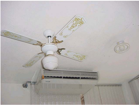
Fig. 15 : Ceiling fan replacing the 1 st Lennox air conditioning unit which does not work and compact low consumption lamp
