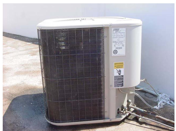
Fig. 20: 2 nd Lennox external unit
